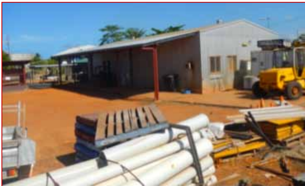
The Council stores area is due for an upgrade which will include a concrete surface, a car park and renovations to the building.
