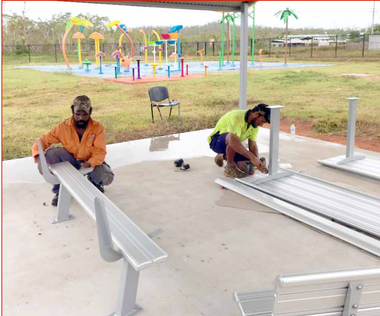
LEFT: Jyren Kyle and Richard Claudie installing new seating at our Splash Park
