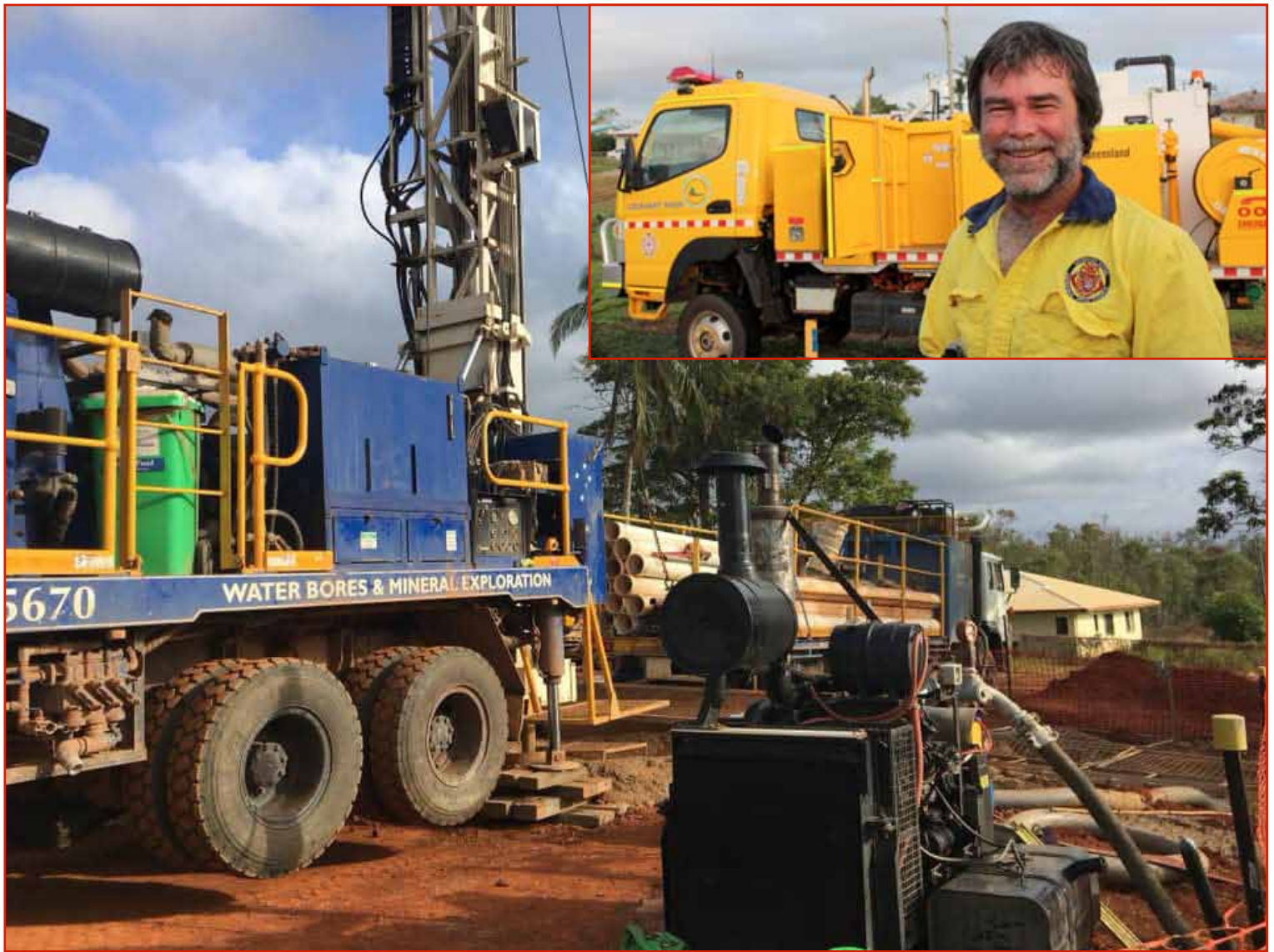
ABOVE: Lockhart River has had some lucky breaks with three extra water bores now in the process of being drilled around town. At least two of those sites have been found to have good quality and plenty of water. Plumber Paul Jensen was back in town for a short visit to help with the development of the new bores pumps, and pipe work as the drilling got underway in early June.
