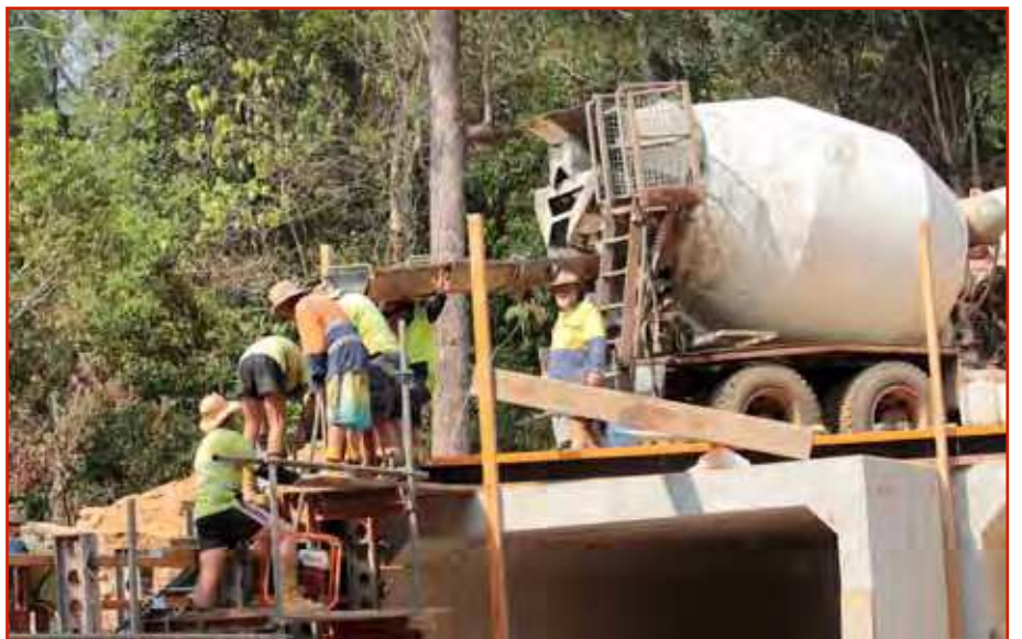
TOP RIGHT: CEO David Clarke ABOVE: concreting the base for the new bridge on the airport/main road.
